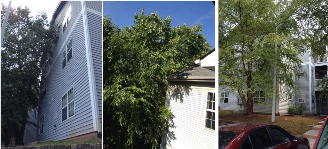
Examples of trees impacting gutters, roofing, and siding
