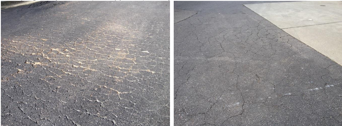
Photos depicting repairs needed at dumpster site near Wolf Tech Lane
