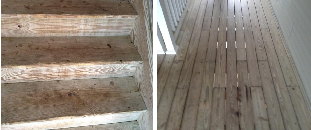
Wooden stairs with treads and risers (left) and wooden decking in breezeways (right)
